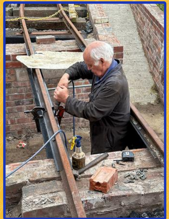
The end is in sight - completion of the new inspection pit draws near, with Paul bolting the rails in place.
