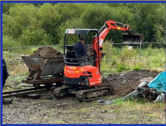
What better job in the pouring rain - moving several tons of earth from the banking at the rear of the site!
